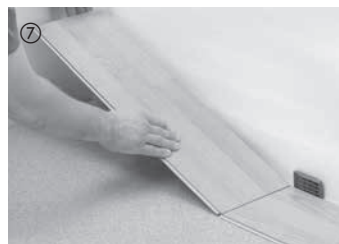
⑦ Cut the last board of the first row to size, leaving an expansion gap of 10--15 mm between the board and wall. Insert the board at a slight angle and rotate it down. The next row is started with the leftover piece of the first row (short side offset of at least 40 cm). This considerably reduces waste.
